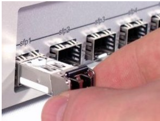
Figure 2.2. Installing a 1000 Base LX/SX module
